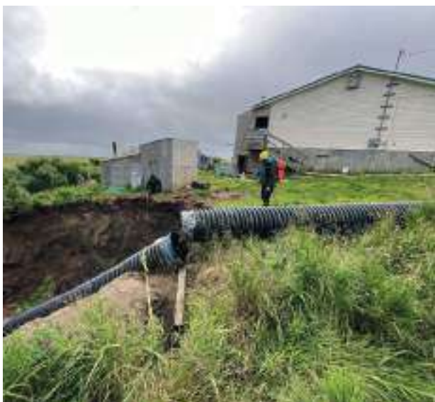
Permafrost thaw contributes to rapid erosion and land destabilization beneath critical community infrastructure in the Alaska Native Village of Cev’aq (Chevak). A massive storm devastated some communities standing on coastal permafrost in southwest Alaska in October 2025.
