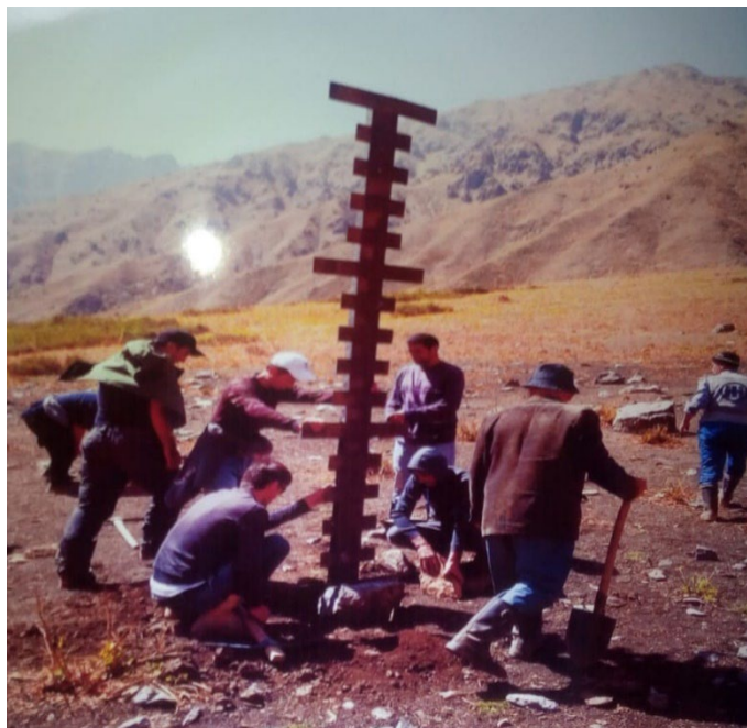
Figure 5. Installation of snow stake in Tajikistan (courtesy of Tajik Hydromet).
